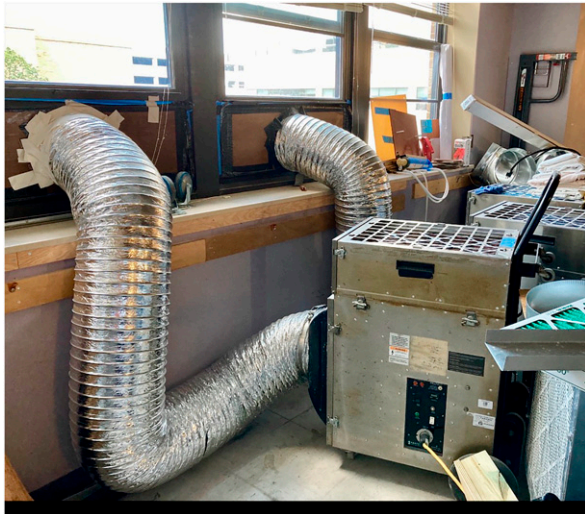
Figure 3. Air scrubbers used to provide negative pressure (units in patients room are usually smaller).
